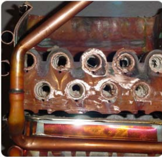
Photo by Rinnai shows scale buildup in the heat exchanger without EasyWater treatment.
